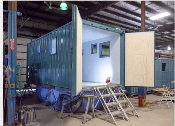
Customized Weatherproof Shipping Container
